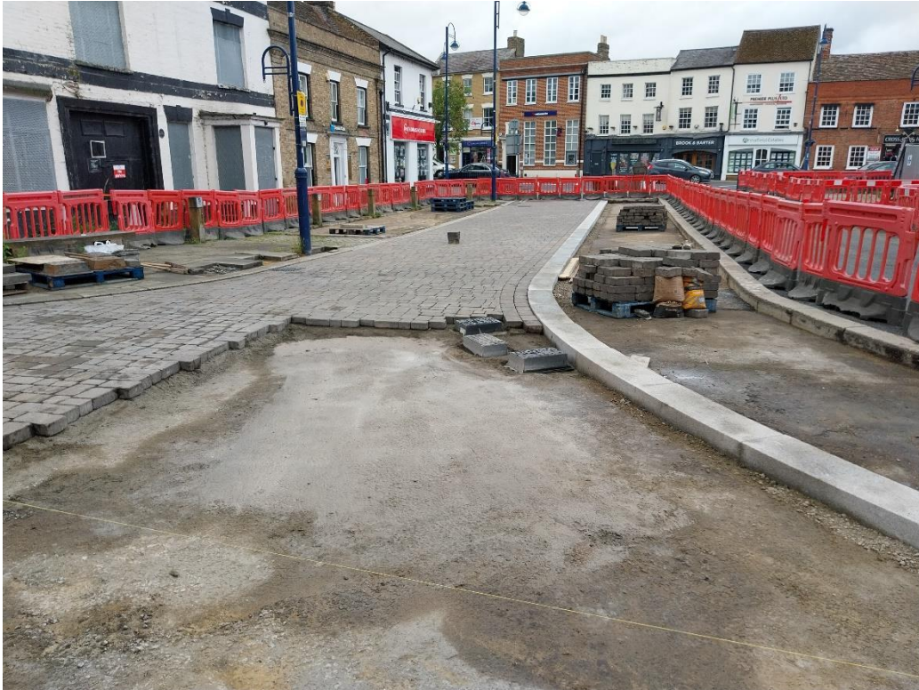
09/07/24 – Relaying of Market Place blockwork continues. A temporary access road is in place to ensure access for residents and businesses at all times.
