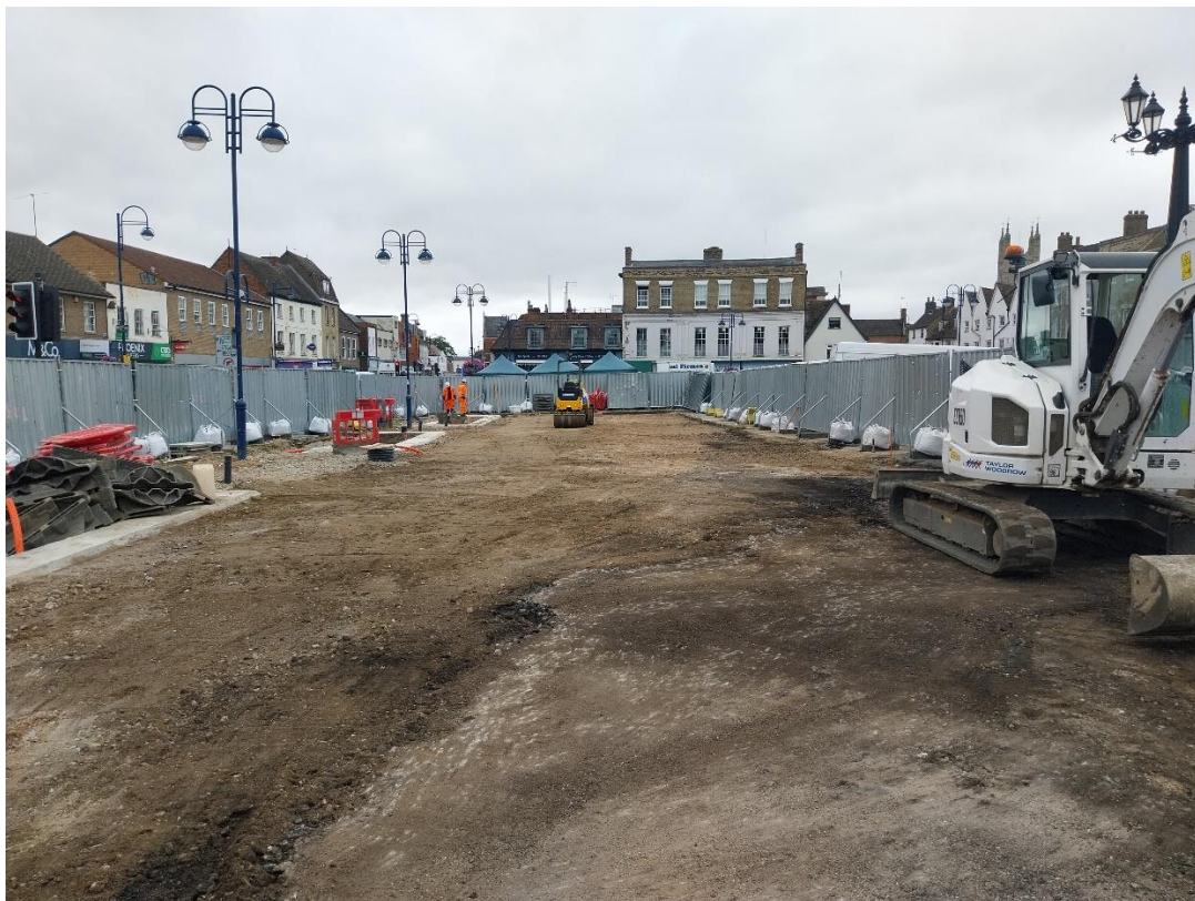
05/09/2024 – Market Square north – SUDS drainage system, electrical ducts and chambers and rain garden foundations all complete. Surface prepared for tarmacking ready for slab laying to commence soon.
