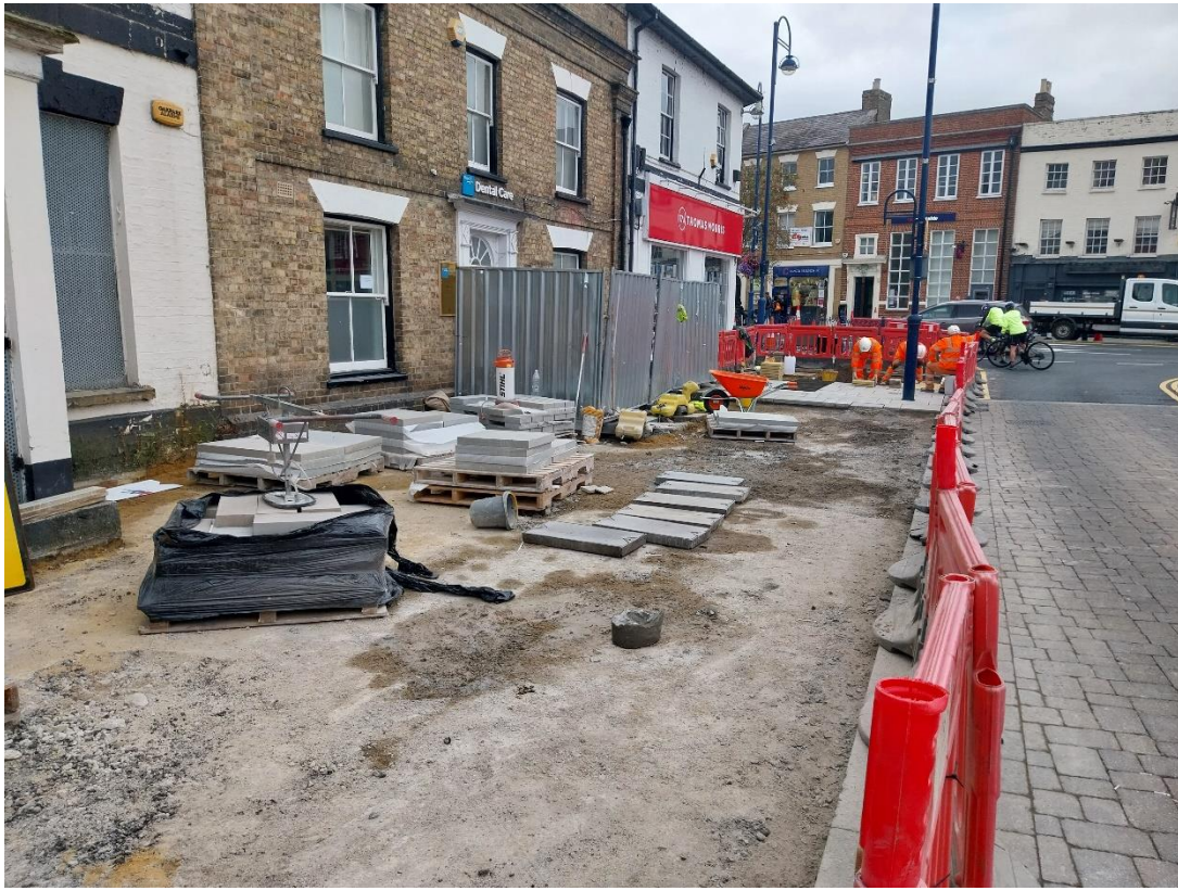
05/09/2024 – Pavement, kerbs and loading bay stripped and repaving commenced outside the Old Falcon
