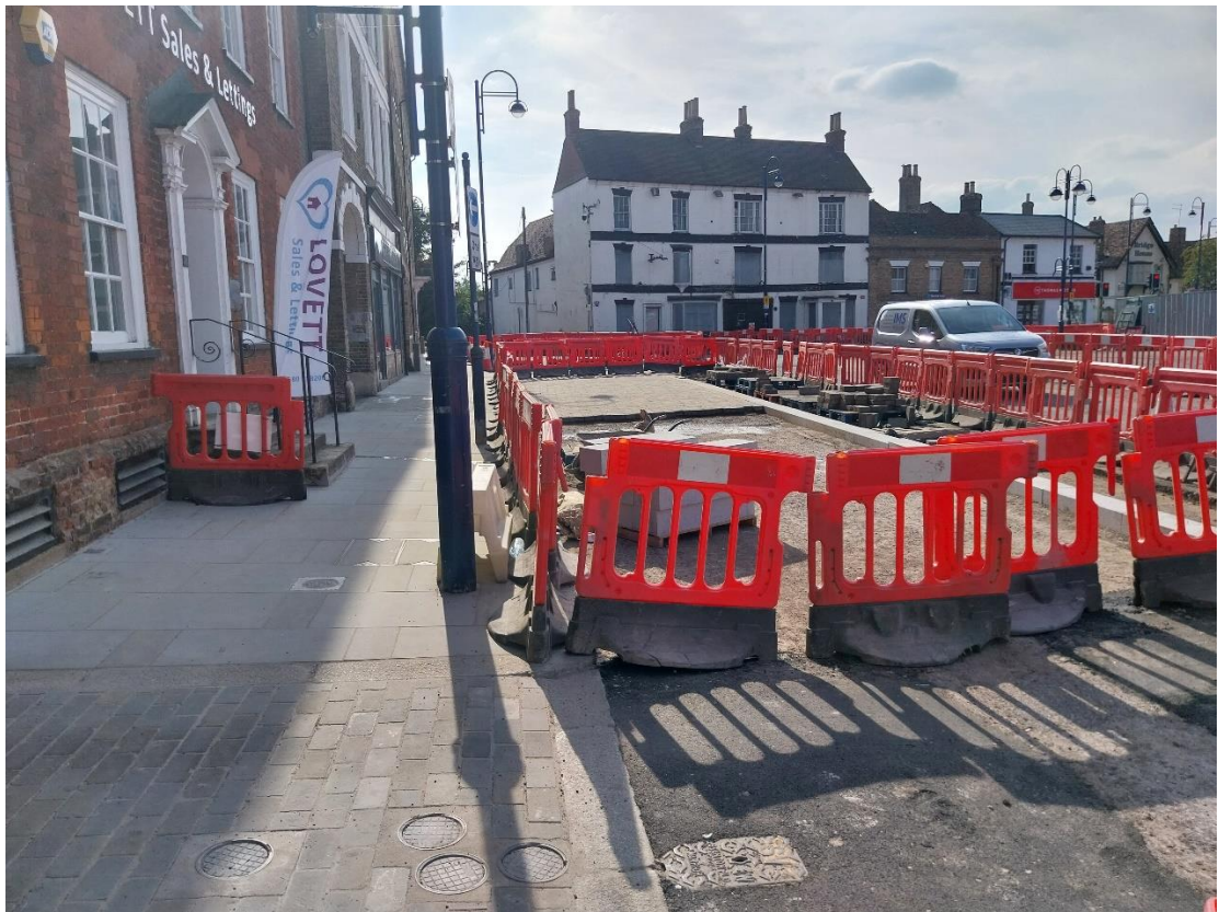
30/07/24 – Footway paving and vehicle access paving complete on South side of Market Square up to the Dogs Trust. Regrading of sub-base and relaying of Market Place blockwork proceeding at pace.
